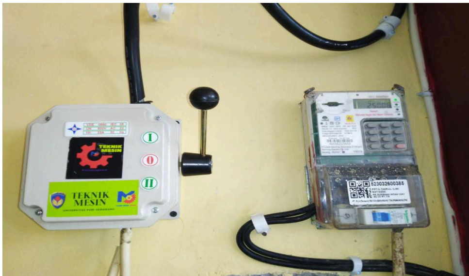
Gb. 1. KWH meter serta handel PLN/Genset
